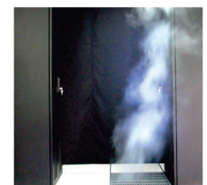
This smoke test shows how the 70° tile forces the smoke toward the cabinet
